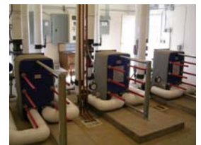
The heat exchangers for the plant are surprisingly compact.
